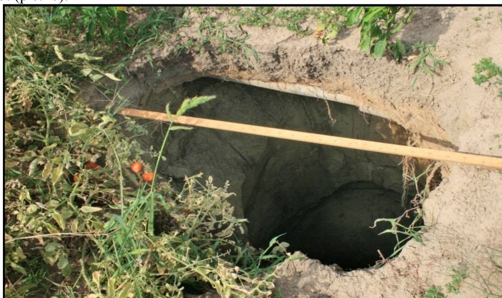
Figure 10 - Failure in the village of Nizhny Baskunchak (Photo by O.M. Vyazmin)
